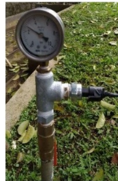
Figure 12. Sensor installation near analog manometer as comparison
