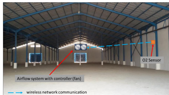
Figure 7. The system layout in the factory.
