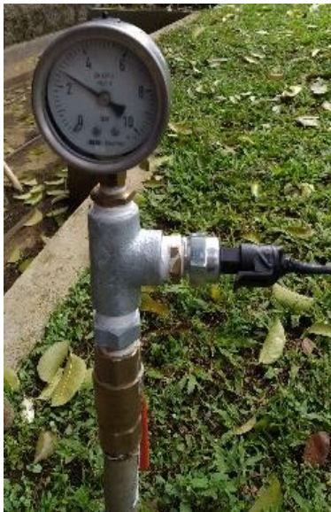
Figure 12. Sensor installation near analog manometer as comparison.
